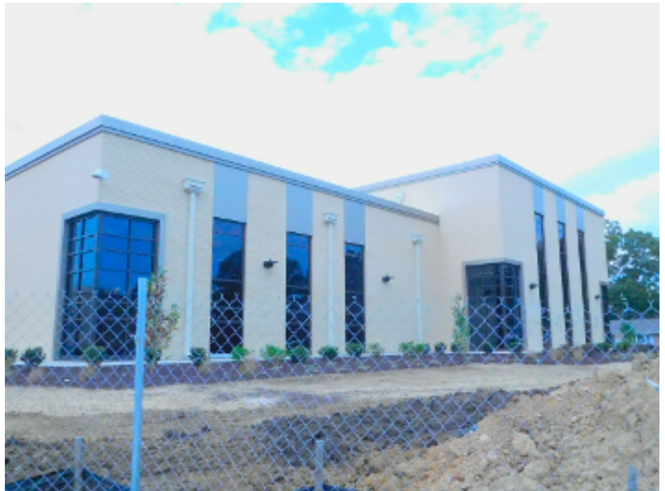
The new fine arts wing will house chorus, band, theater, art and health classes. Currently these classes are being held in various locations in the main building and in the tech center. The teachers are looking forward to being reunited as a department when this new addition opens.
